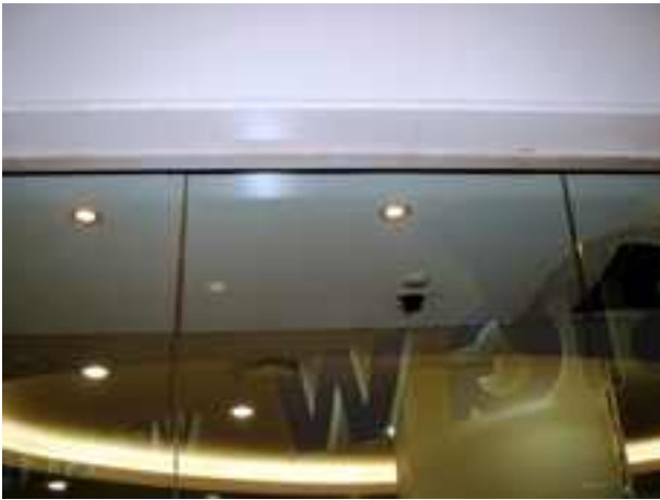
THE BLOB? NO, IT'S SUPPOSED TO BE WATERPROOFING
