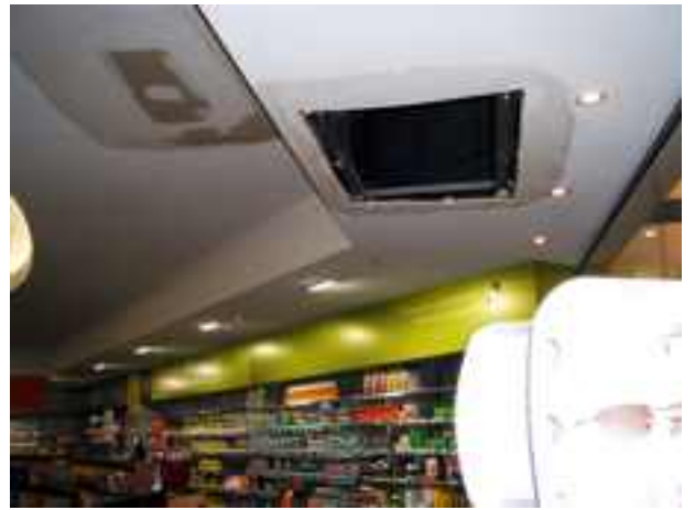
NEW PATCHES NEW WATER LEAKS SHOWING
