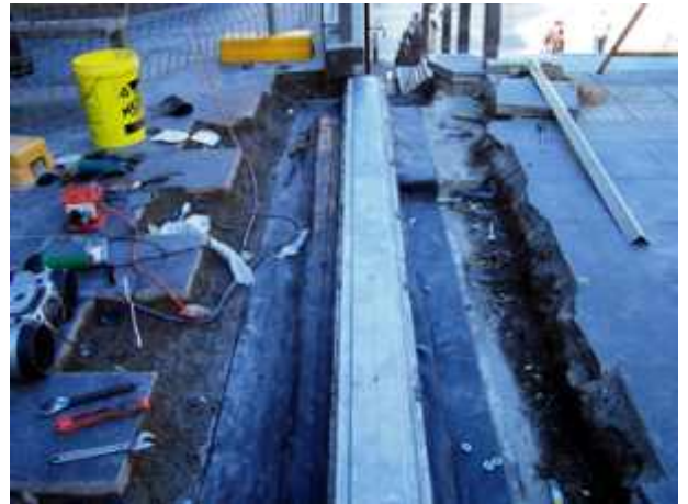
WE HAD TO CONTINUE DOWN THE STEPS TO FOLLOW THE CONSTRUCTION JOINT
